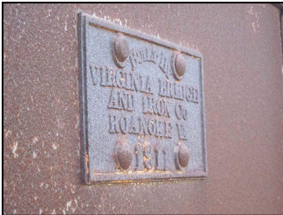
View Northwest, Plate on North End of West Girder. Reads "BUILT BY / VIRGINIA BRIDGE / AND IRON Co / ROANOKE VA / 1911 (WVDOH March 18, 2014)
