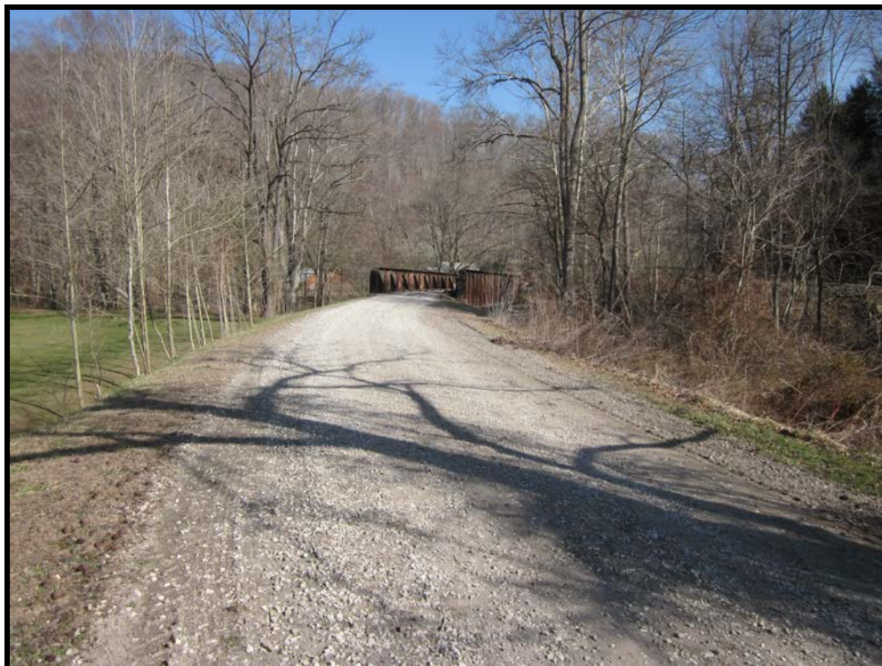
View North/Northwest, Looking Toward South Approach to Fleming Thru Girder Bridge (WVDOH March 18, 2014).
