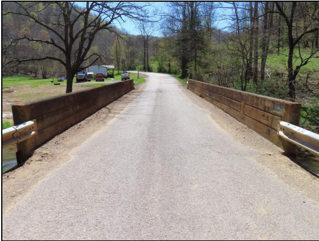
North Approach. View SE (WVDOH 4/17/2025). North End of Downstream/West Railing has County Plaque.
