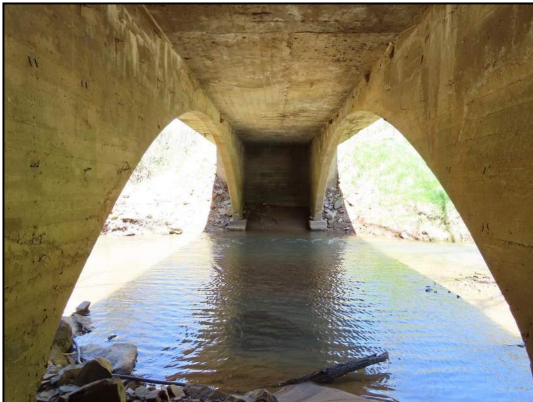
Spandrel Walls, North Abutment, and Underside of Deck. View NW, taken from South Abutment (WVDOH 4/17/2025)
