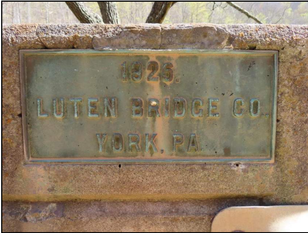
Bridge Builder's Plaque at South End of Upstream/East Railing. View NE (WVDOH 4/17/2025)
