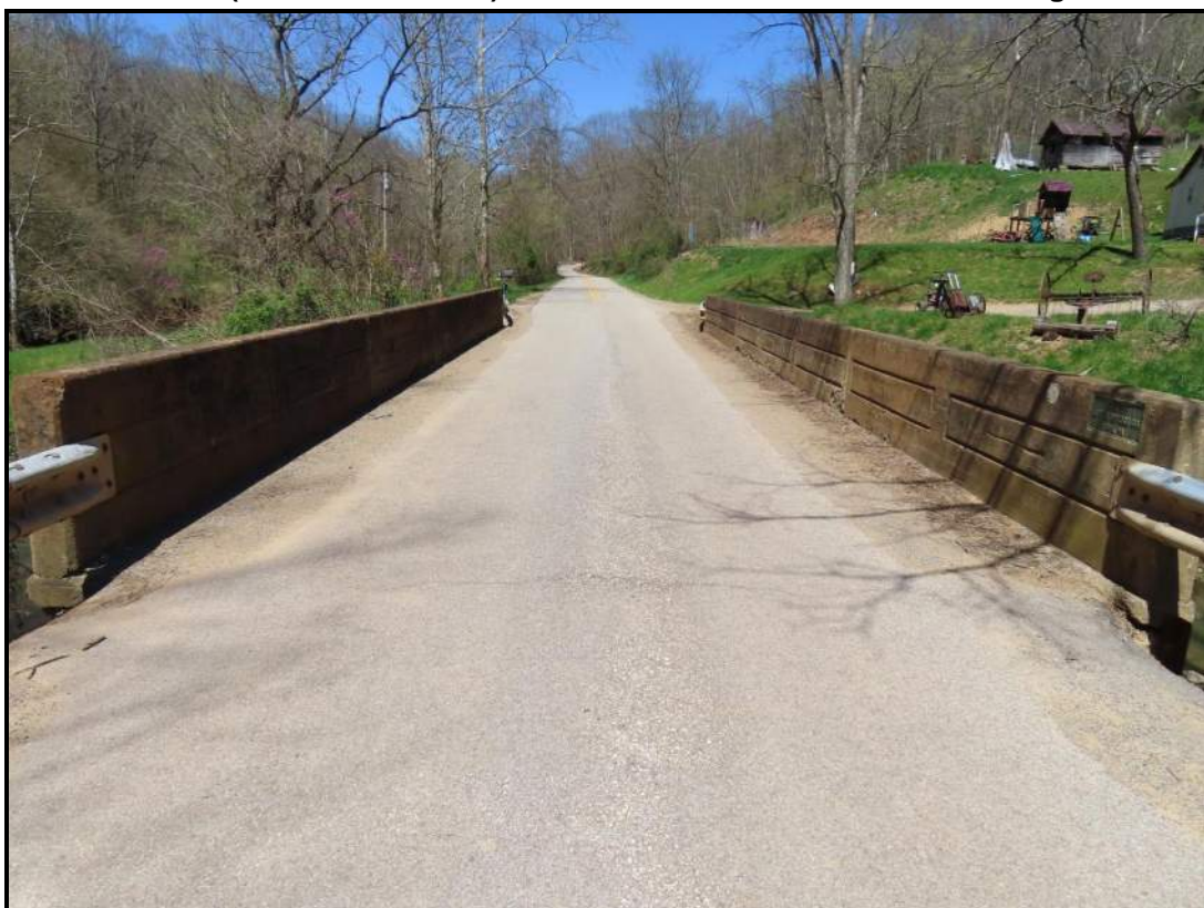
South Approach. View NW (WVDOH 4/17/2025). South End of Upstream/East Railing has Builder's Plaque.
