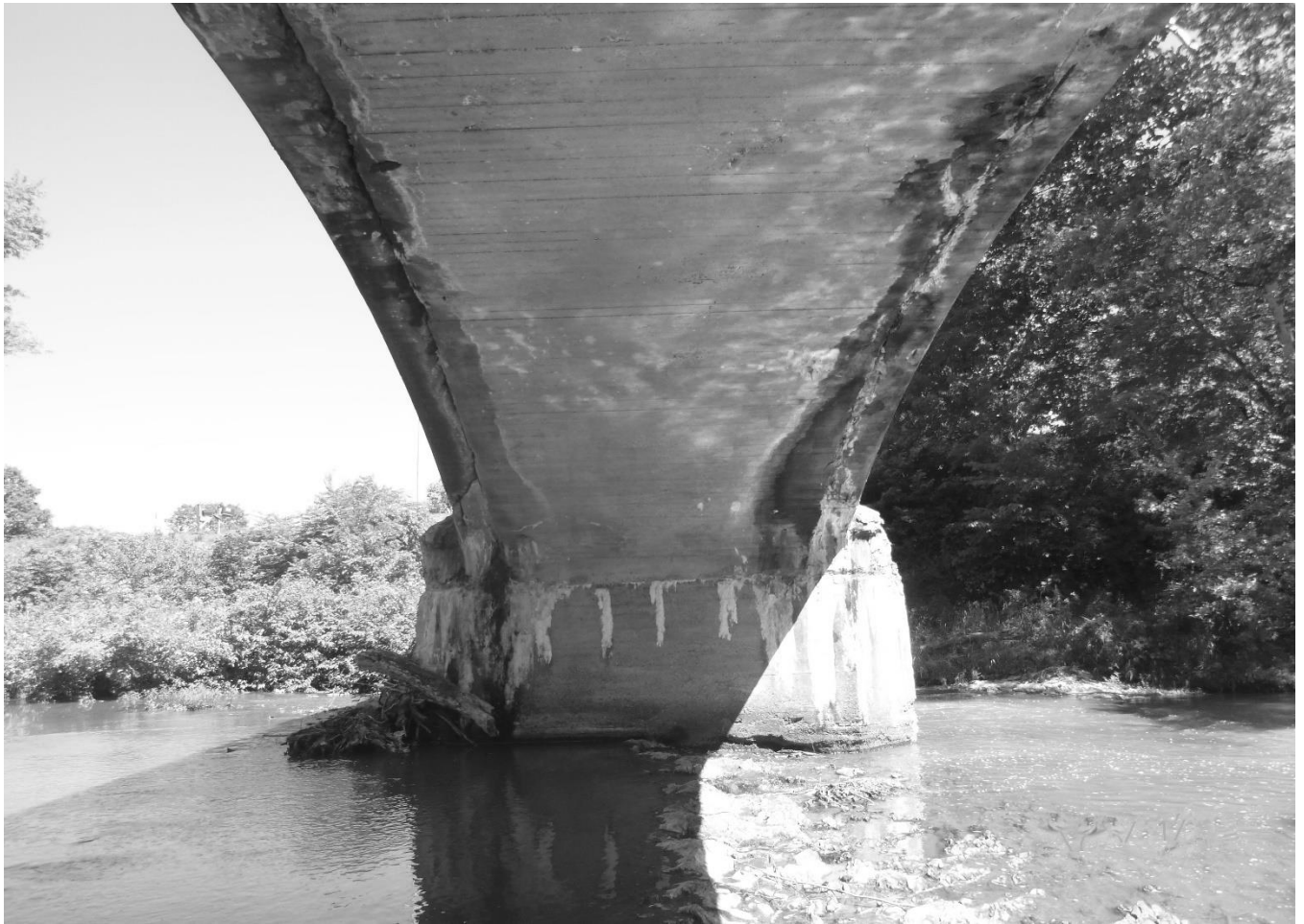
Photo 6 Charles Milar Bridge Mineral County County Route 10 spanning Patterson Creek View of pier
