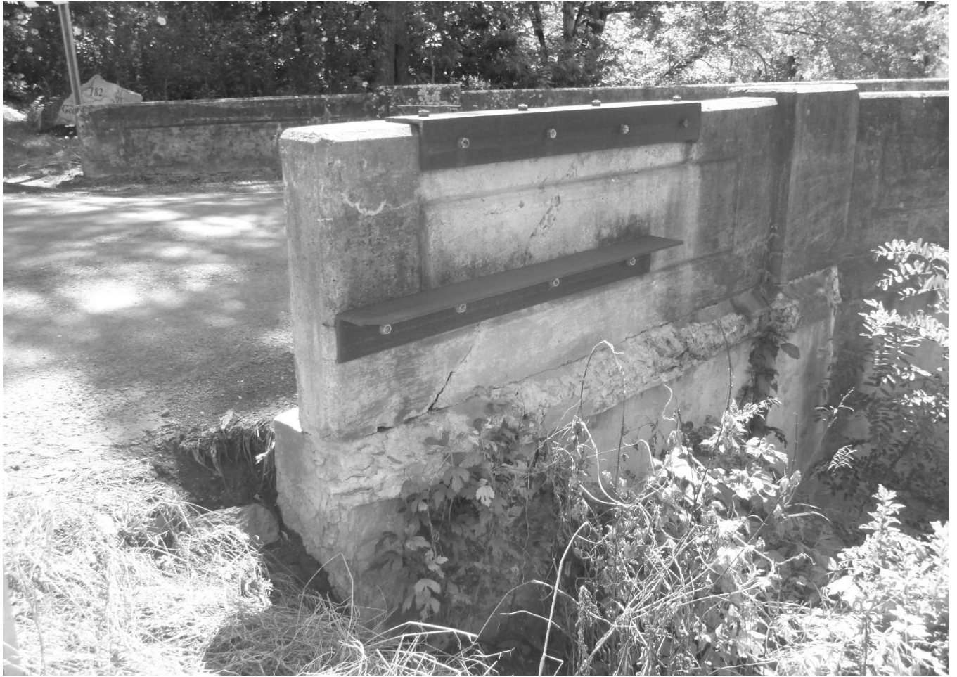
Photo 9 Charles Milar Bridge Mineral County County Route 10 spanning Patterson Creek Repair to north parapet corner of west abutment
