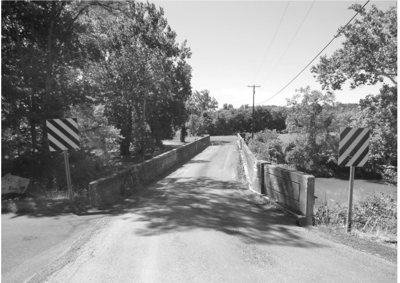
Photo 1 Charles Milar Bridge Mineral County County Route 10 spanning Patterson Creek North approach to bridge, view south
