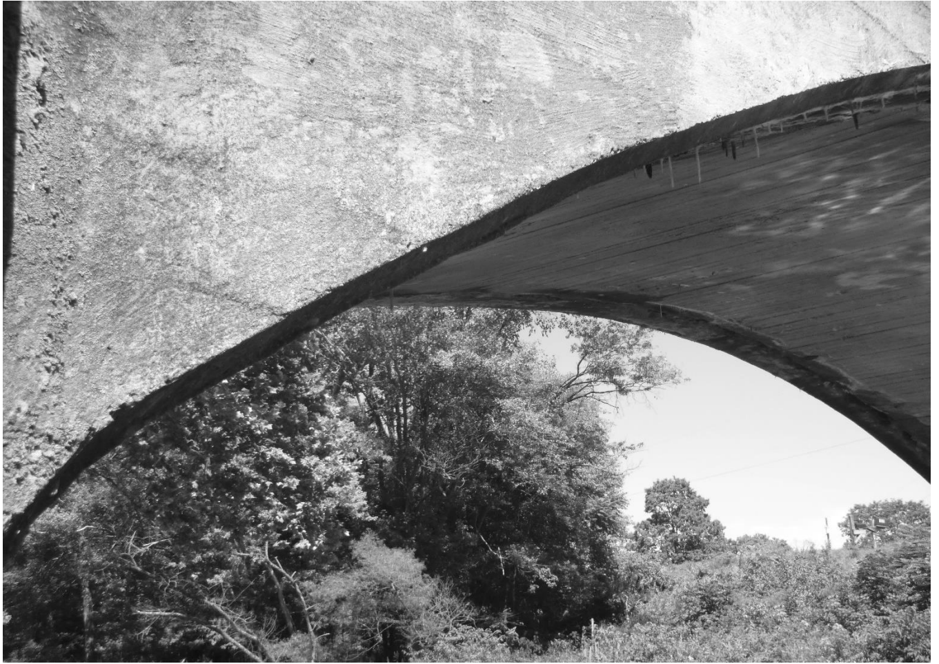
Photo 12 Charles Milar Bridge Mineral County County Route 10 spanning Patterson Creek Detail of arch ring
