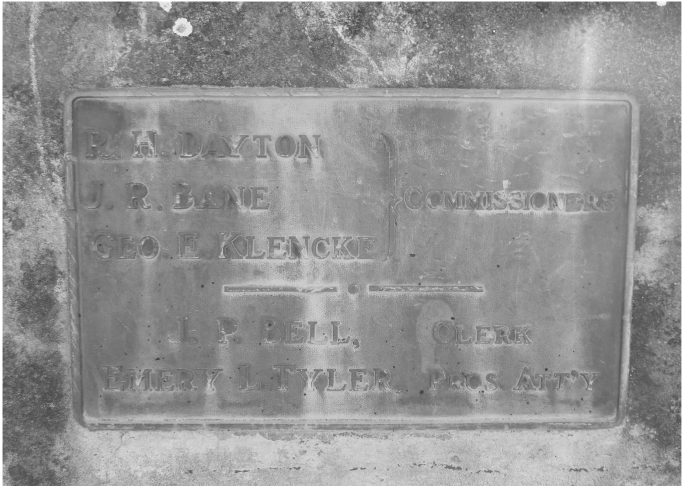
Photo 7 Charles Milar Bridge Mineral County County Route 10 spanning Patterson Creek Metal plaque on west parapet
