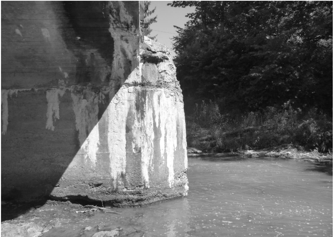
Photo 11 Charles Milar Bridge Mineral County County Route 10 spanning Patterson Creek Detail of pier and nose
