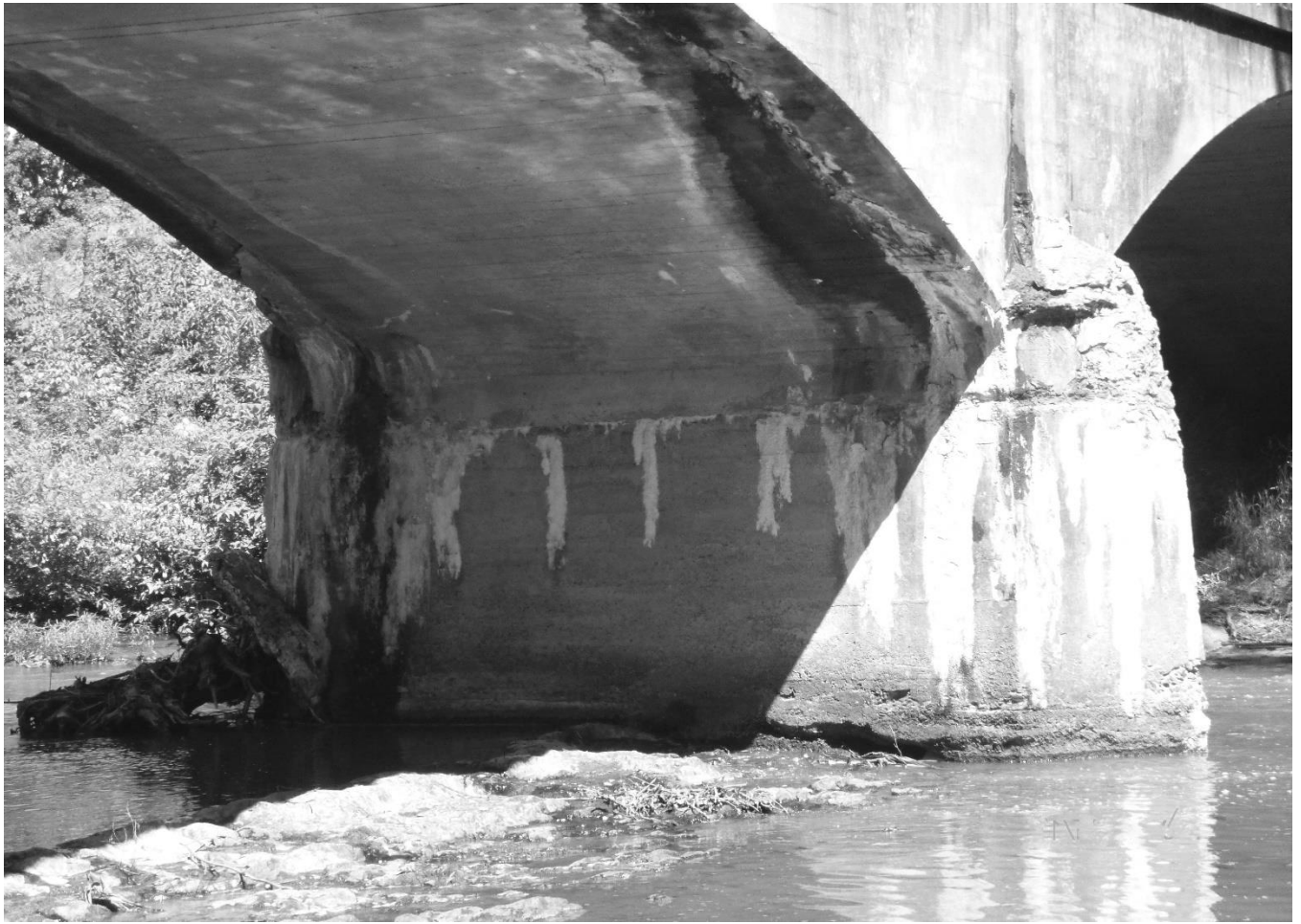
Photo 10 Charles Milar Bridge Mineral County County Route 10 spanning Patterson Creek Center pier
