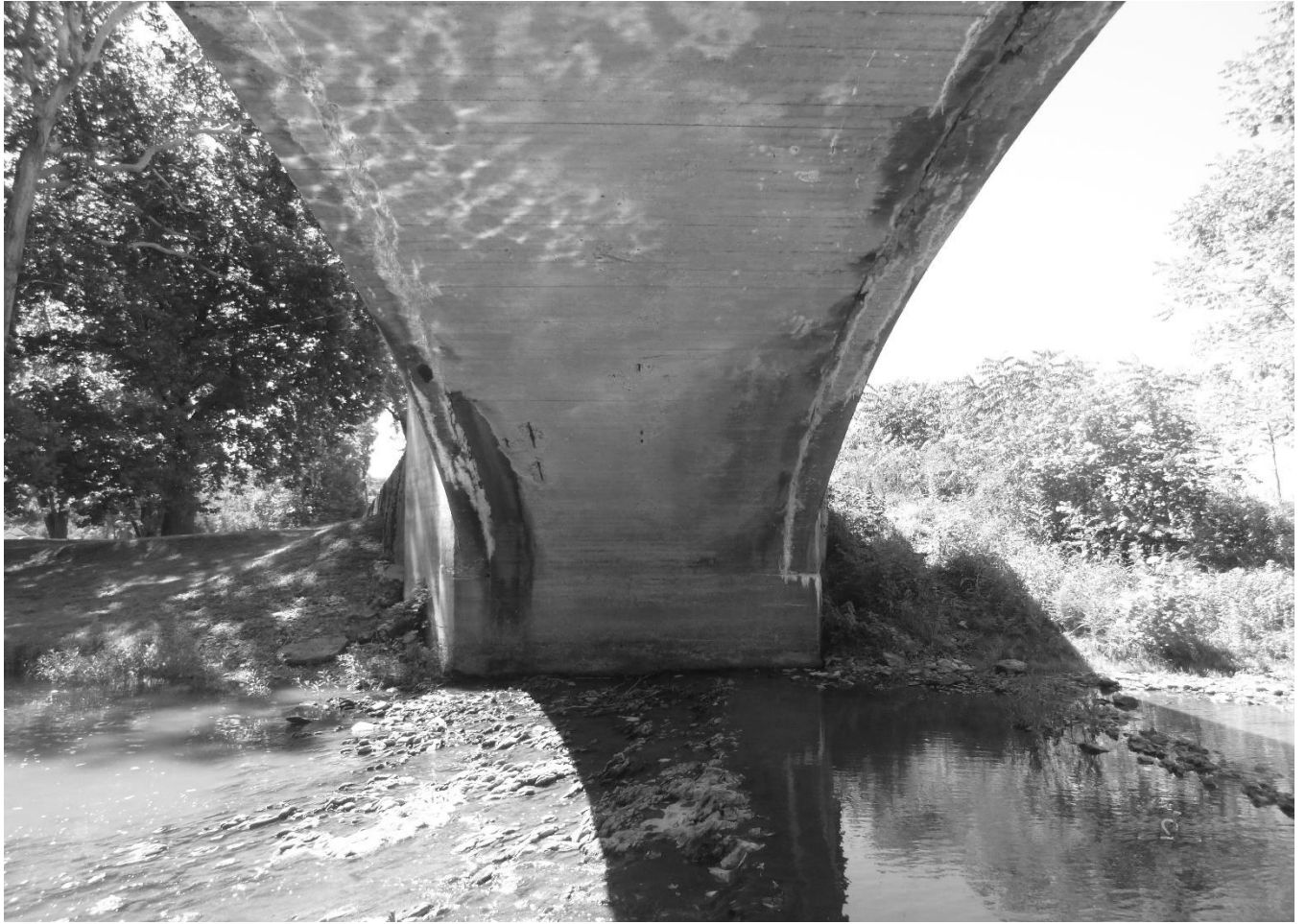
Photo 5 Charles Milar Bridge Mineral County County Route 10 spanning Patterson Creek View of south abutment
