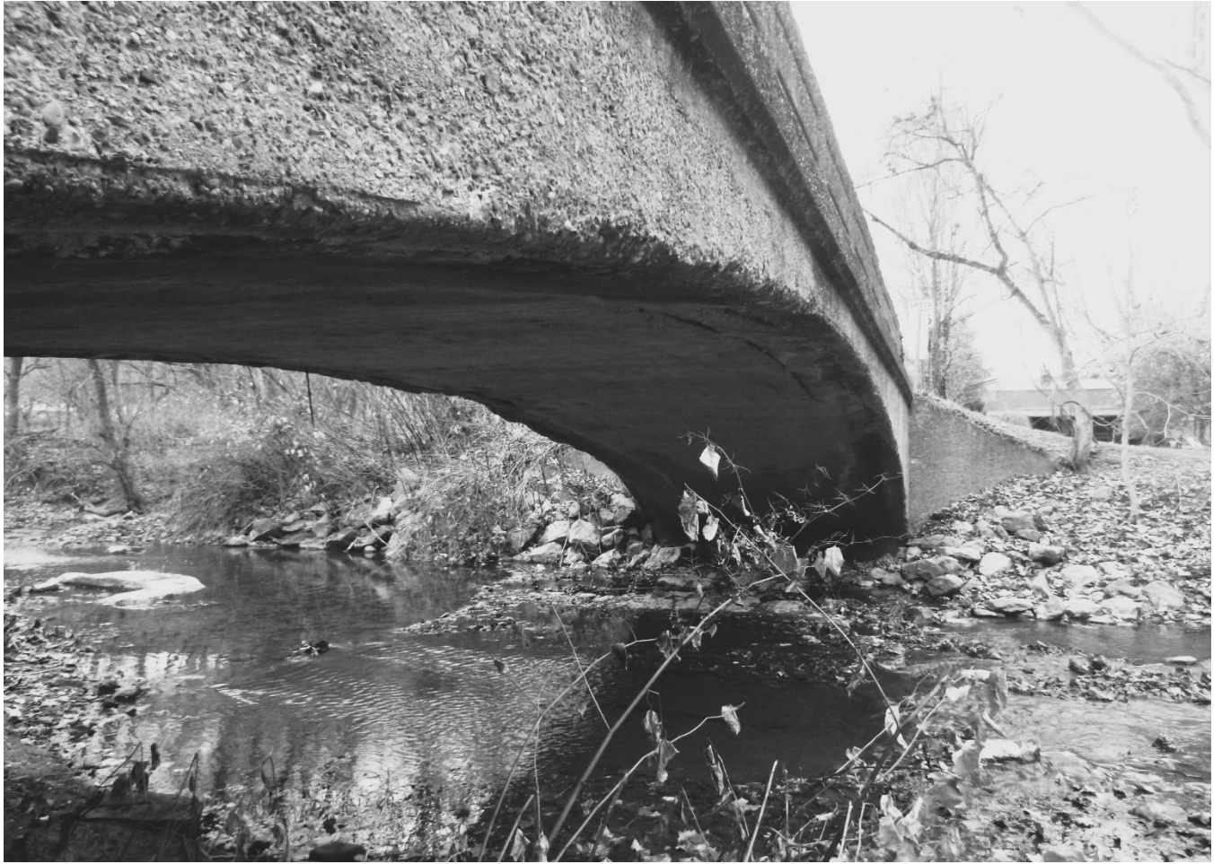
Photo 6 Log Cabin Bridge Brooke County County Route 1/3 spanning Harmon Creek View of north abutment and arch barrel
