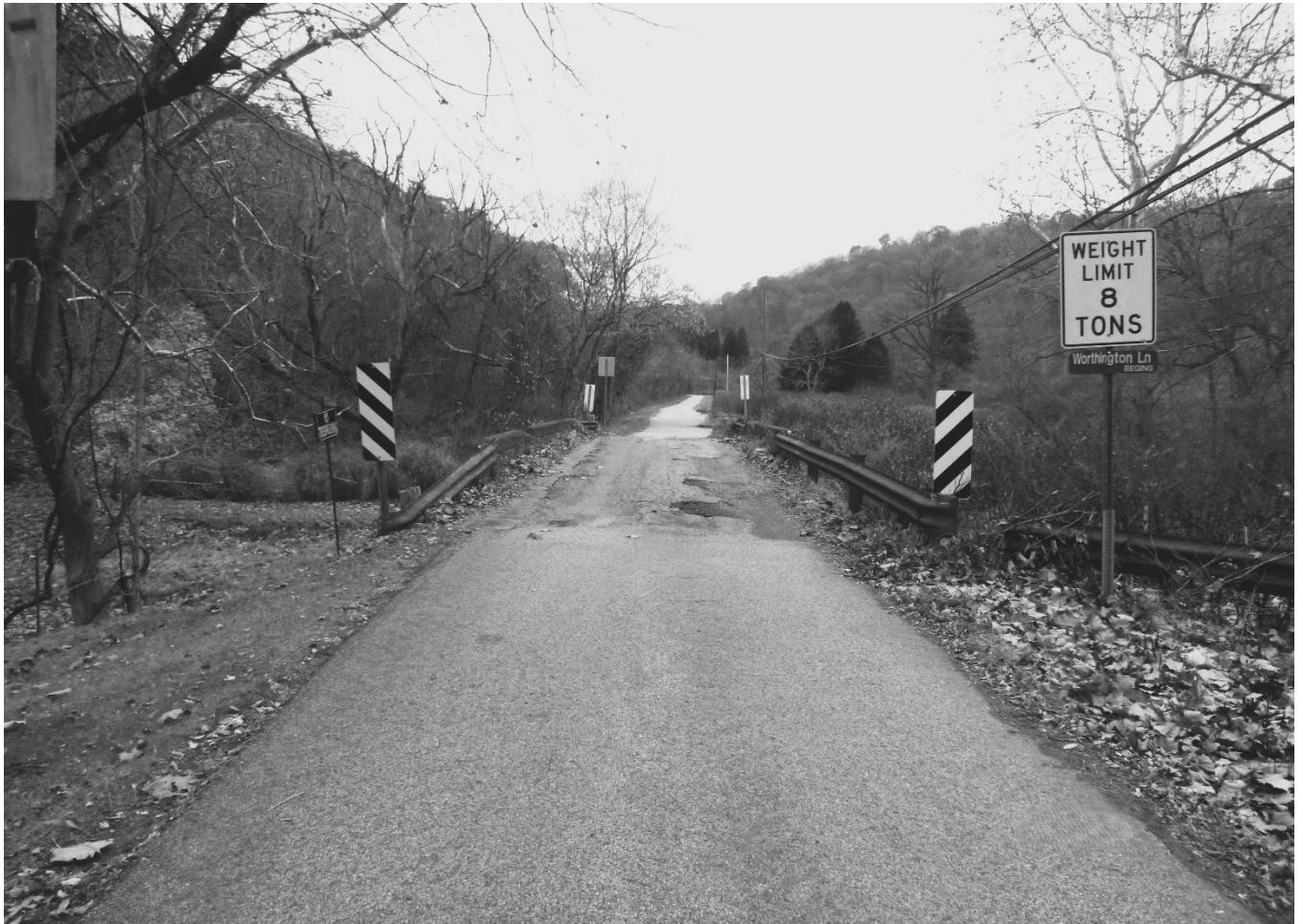
Photo 2 Log Cabin Bridge Brooke County County Route 1/3 spanning Harmon Creek North approach to bridge, view south
