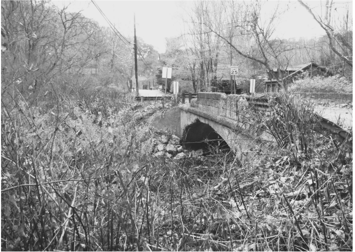
Photo 4 Log Cabin Bridge Brooke County County Route 1/3 spanning Harmon Creek Upstream elevation, view from south foot
