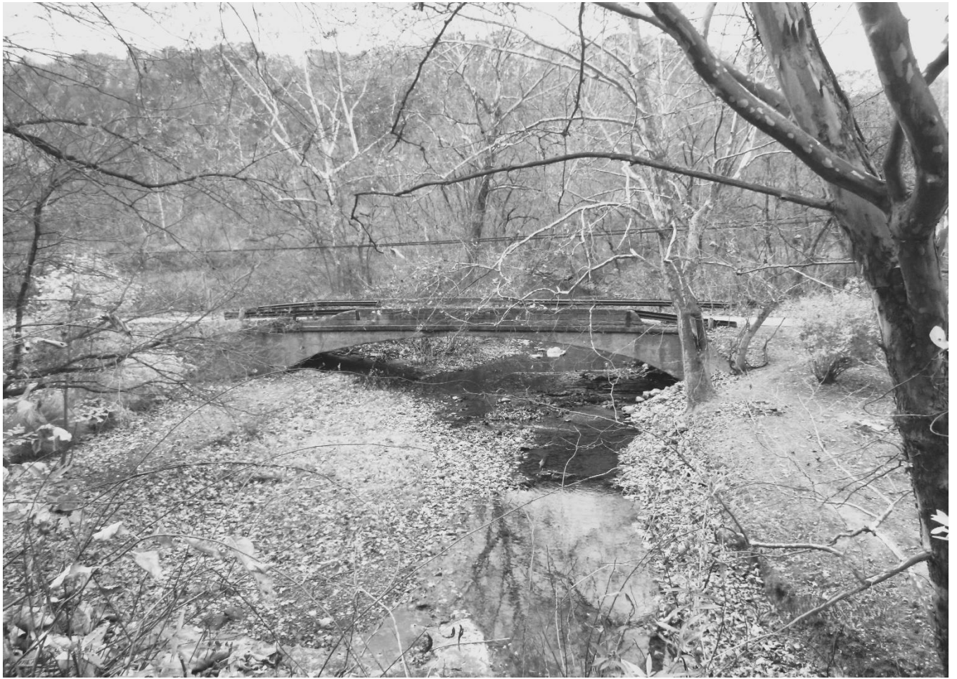
Photo 7 Log Cabin Bridge Brooke County County Route 1/3 spanning Harmon Creek Downstream elevation
