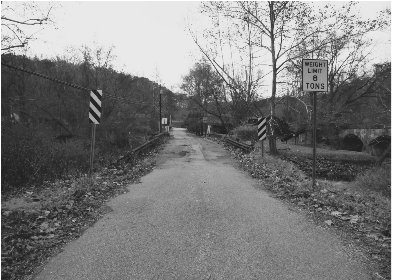
Photo 1 Log Cabin Bridge Brooke County County Route 1/3 spanning Harmon Creek South approach to bridge, view north
