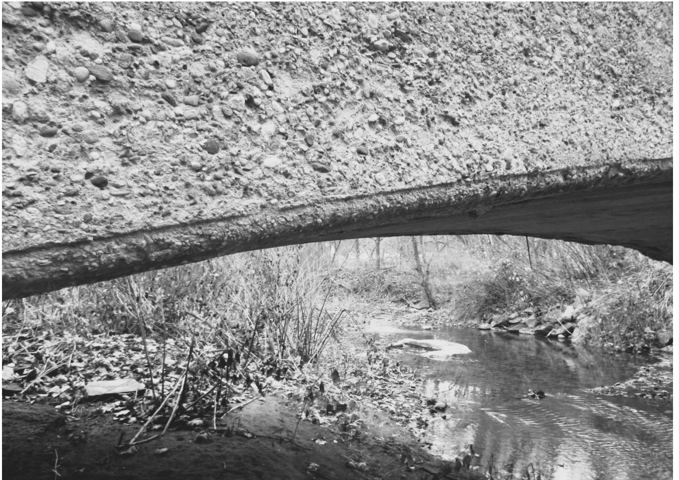
Photo 5 Log Cabin Bridge Brooke County County Route 1/3 spanning Harmon Creek Detail of arch ring with typical Luten rounded edge
