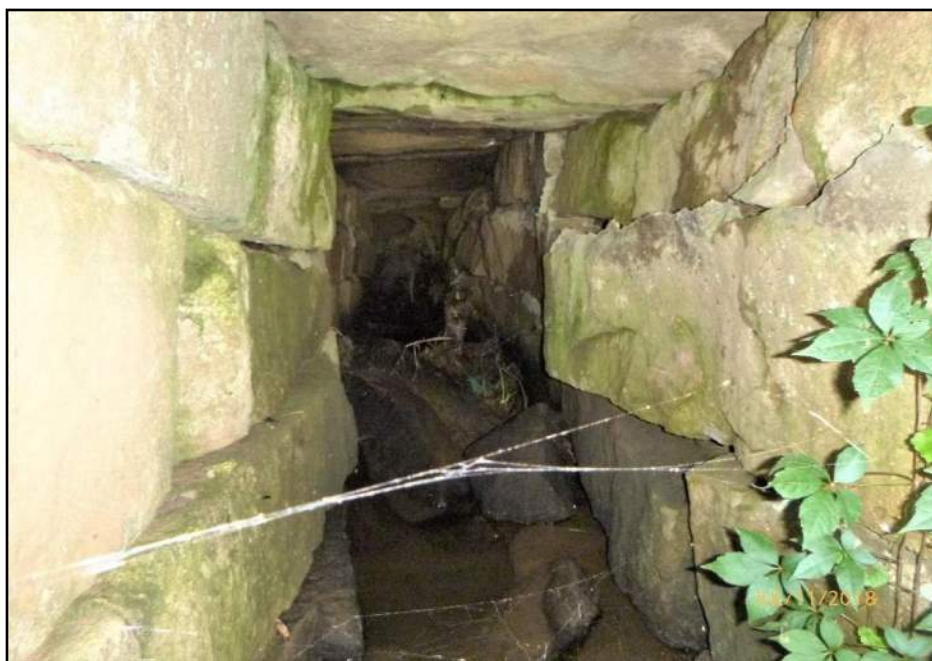
Culvert interior (lightened photo) Blocks on ground are likely from the demolition of the north inlet.
