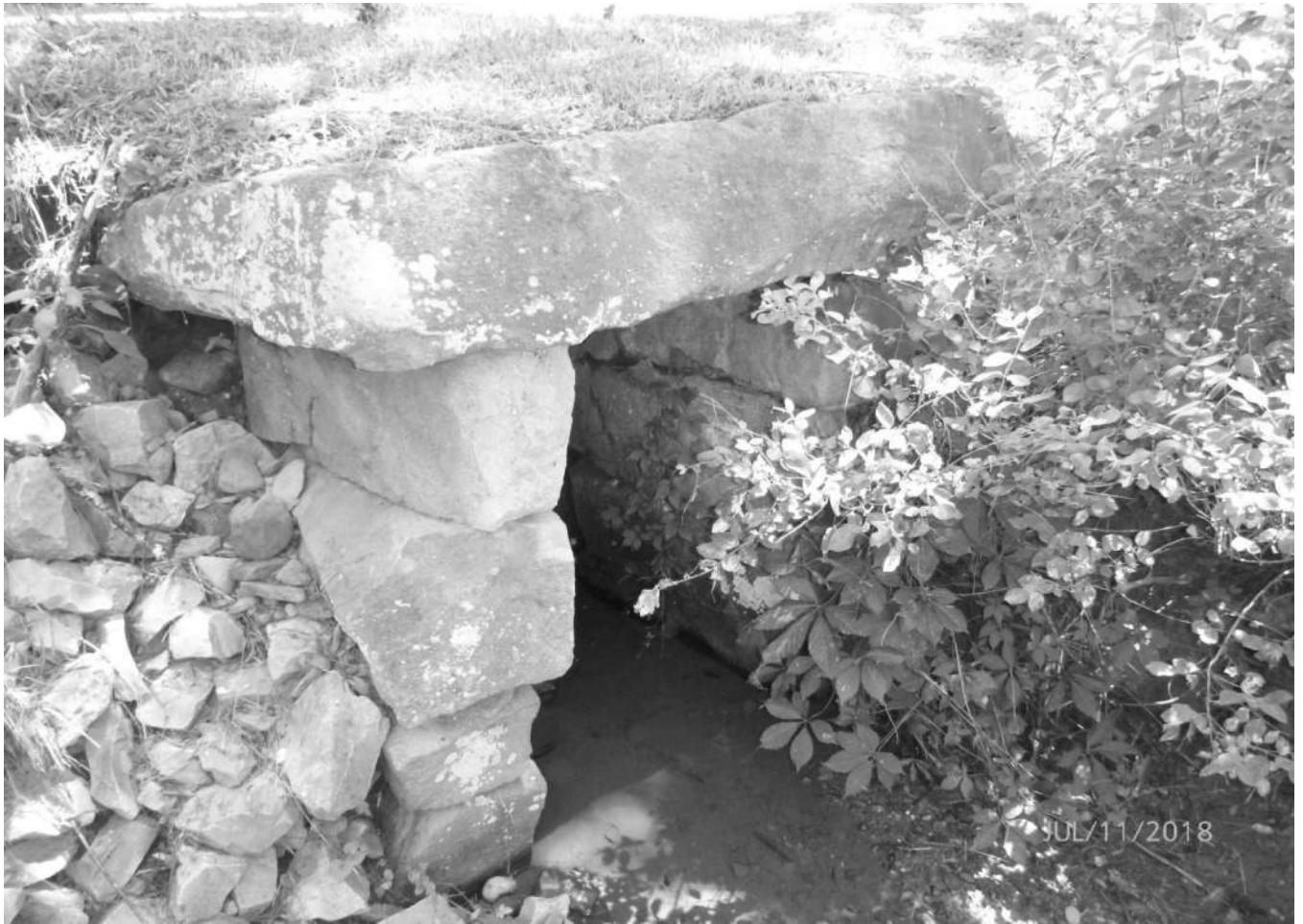
Photo 6 Hallsburg Road Culvert Clay County County Route 42 over tributary of Big Otter Creek Elevation view
