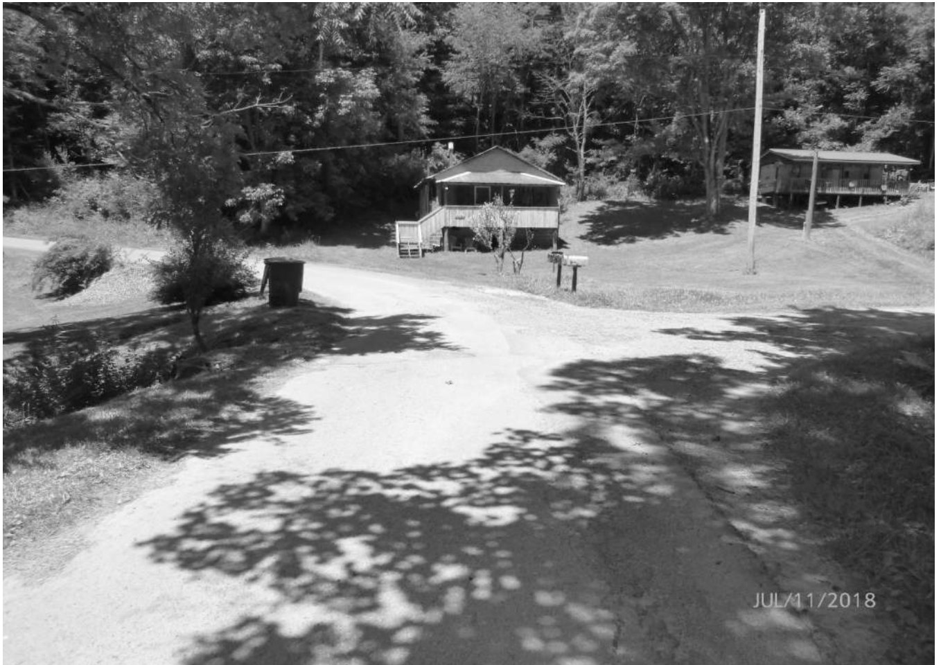
Photo 2 Hallsburg Road Culvert Clay County County Route 42 over tributary of Big Otter Creek North approach to culvert
