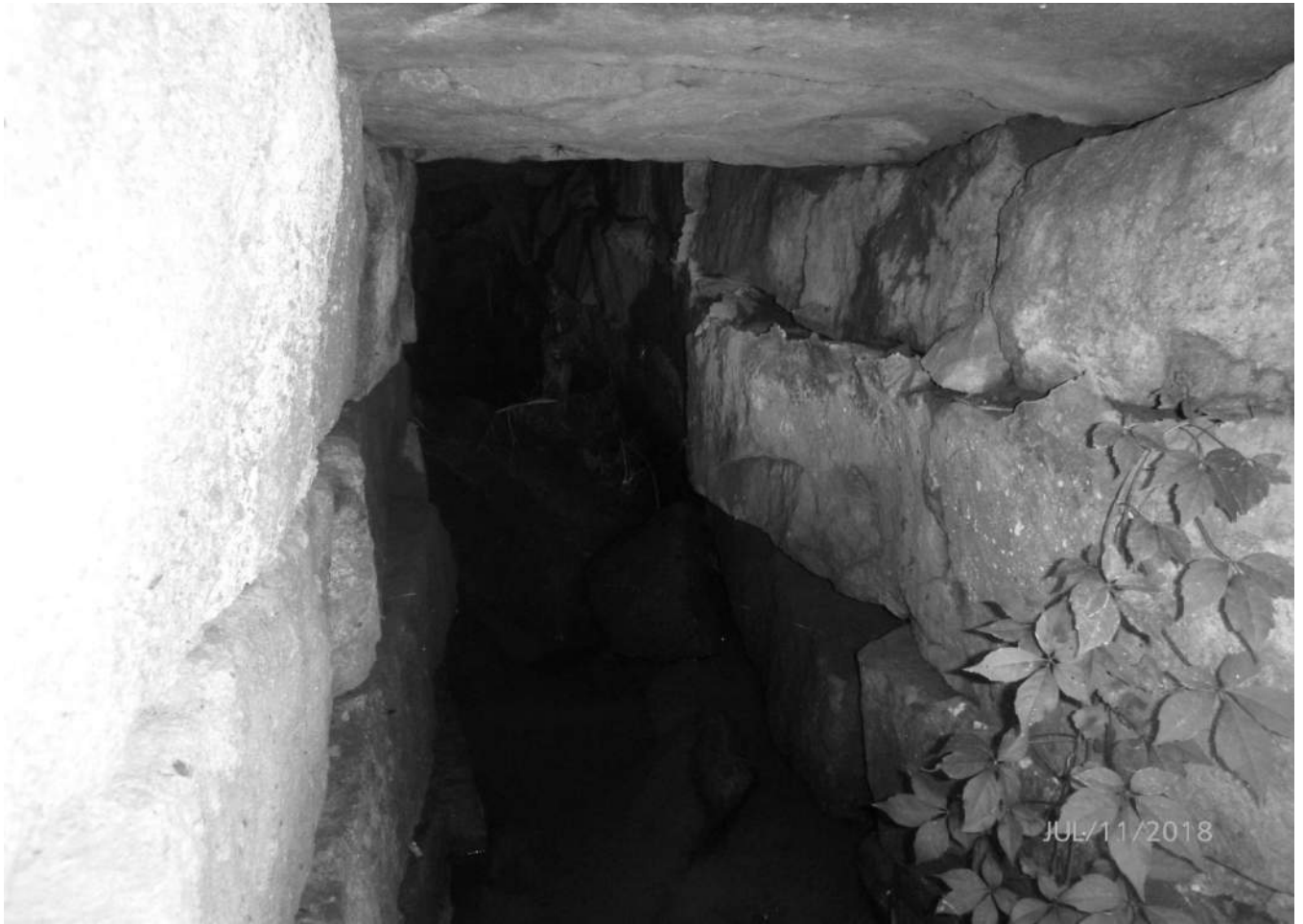
Photo 5 Hallsburg Road Culvert Clay County County Route 42 over tributary of Big Otter Creek Interior view of culvert
