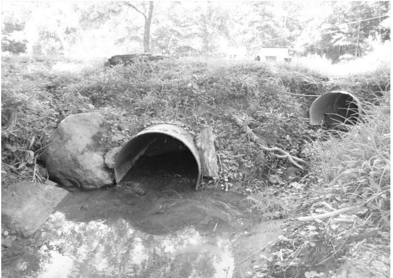
Photo 4 Hallsburg Road Culvert Clay County County Route 42 over tributary of Big Otter Creek Culvert inlet
