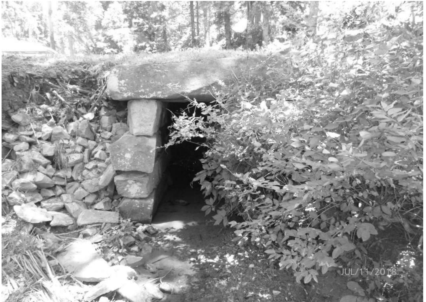
Photo 3 Hallsburg Road Culvert Clay County County Route 42 over tributary of Big Otter Creek Culvert outlet
