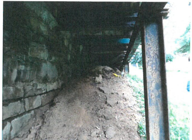
Fill material over southern end of wall & metal support beams & concrete coping added to wall. (2016)
